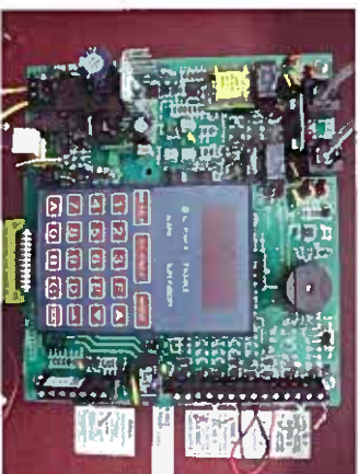
Looking at board enclosed in the back-box.
